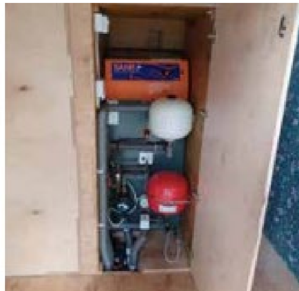
Hot water system
